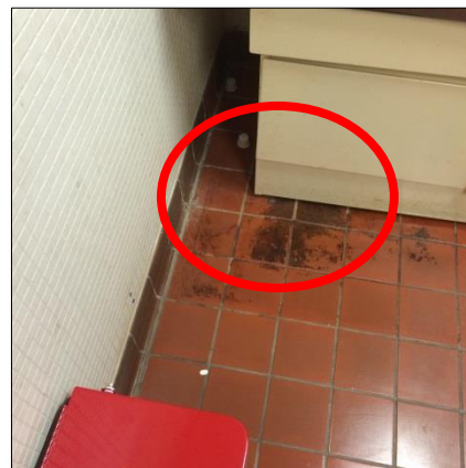
Figure 1: Dirt on exam room floor
