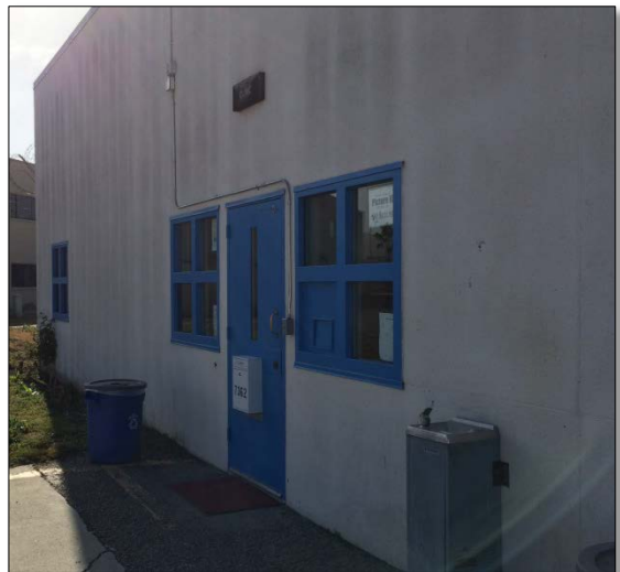
Figure 3: Insufficient protection from inclement weather
