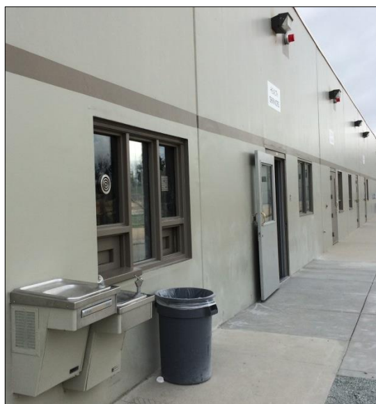
Figure 3: Medication line window without protection for patients from inclement weather
