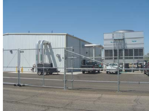
Figure 1 - CVSP's new chiller plant used for inmate housing air-conditioning
