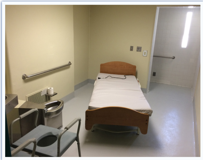
Photo 7. Recently completed health care facility improvement program room unable to accommodate an ADA patient (view 1, photographed 6/10/19).
