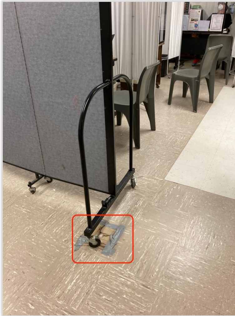
Photo 11. Damaged and unsanitary examination room floor (photographed on 2-14-23).
