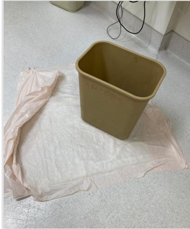
Photo 6. Medication distribution room with ongoing water leak issues (photographed on 6-6-23).
