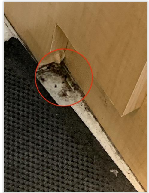
Photo 11. Unsanitary medical room floor (photographed on 9-26-23).
