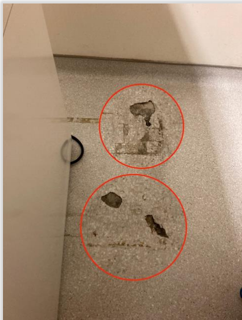
Photo 12. Damaged and unsanitary examination room floor (photographed on 9-28-23).
