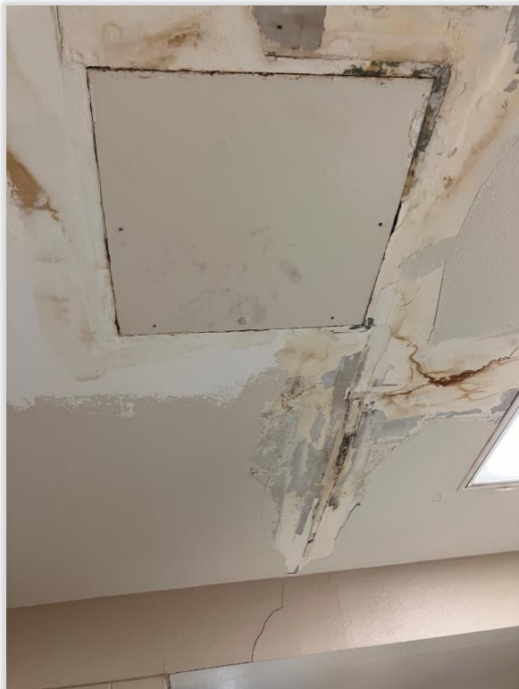
Photo 6. Ceiling damage in the receiving and release area (photographed on 11-28-23).
