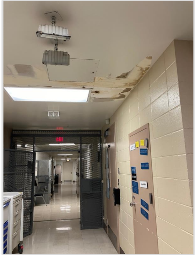
Photo 5. Ceiling damage in the outpatient housing unit (photographed on 11-30-23).
