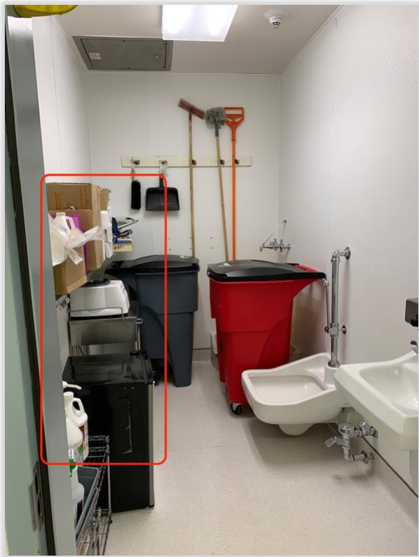
Photo 8. Laboratory equipment and supplies stored in the soiled utility room (photo 2 of 3, photographed on 10-24-23).
