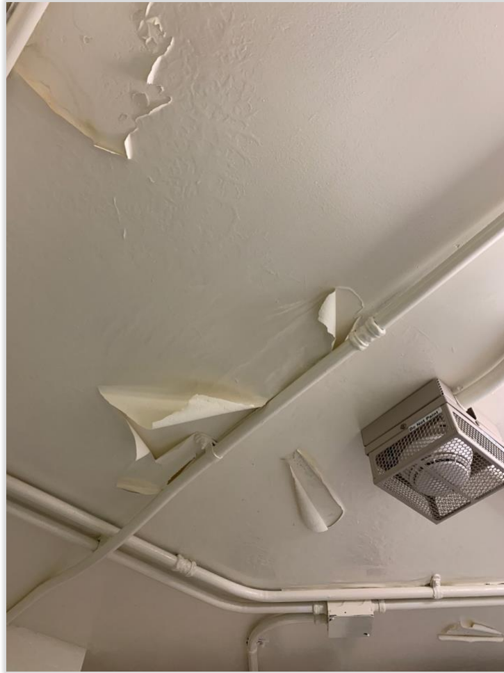
Photo 10. Peeling paint on the clinic ceiling (photographed on 10-25-23).
